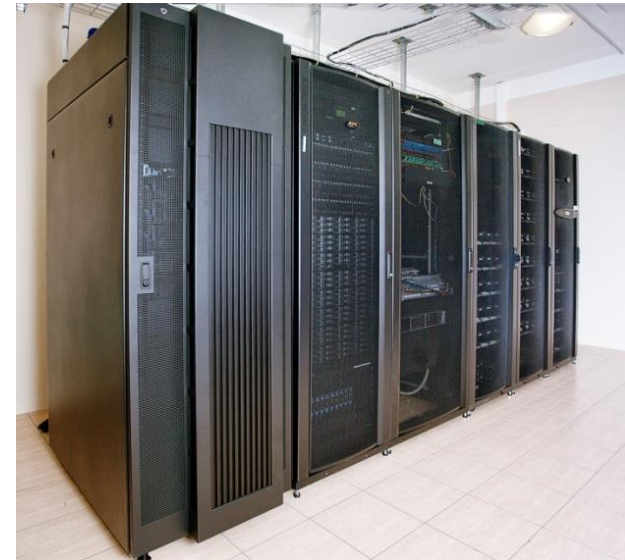
Shared Facility Centre 'Data Centre of FEB RAS' (Khabarovsk, Russia)
